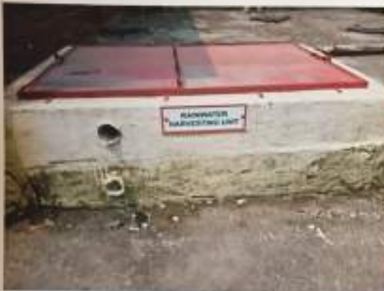
Rainwater Harvesting Unit
