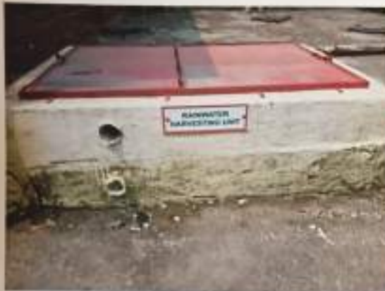
Rainwater Harvesting Unit
