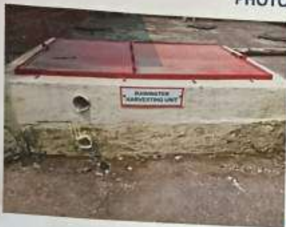
Rainwater Harvesting Unit
