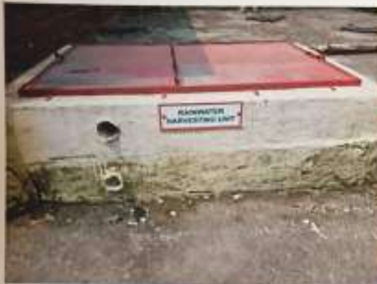
Rainwater Harvesting Unit
