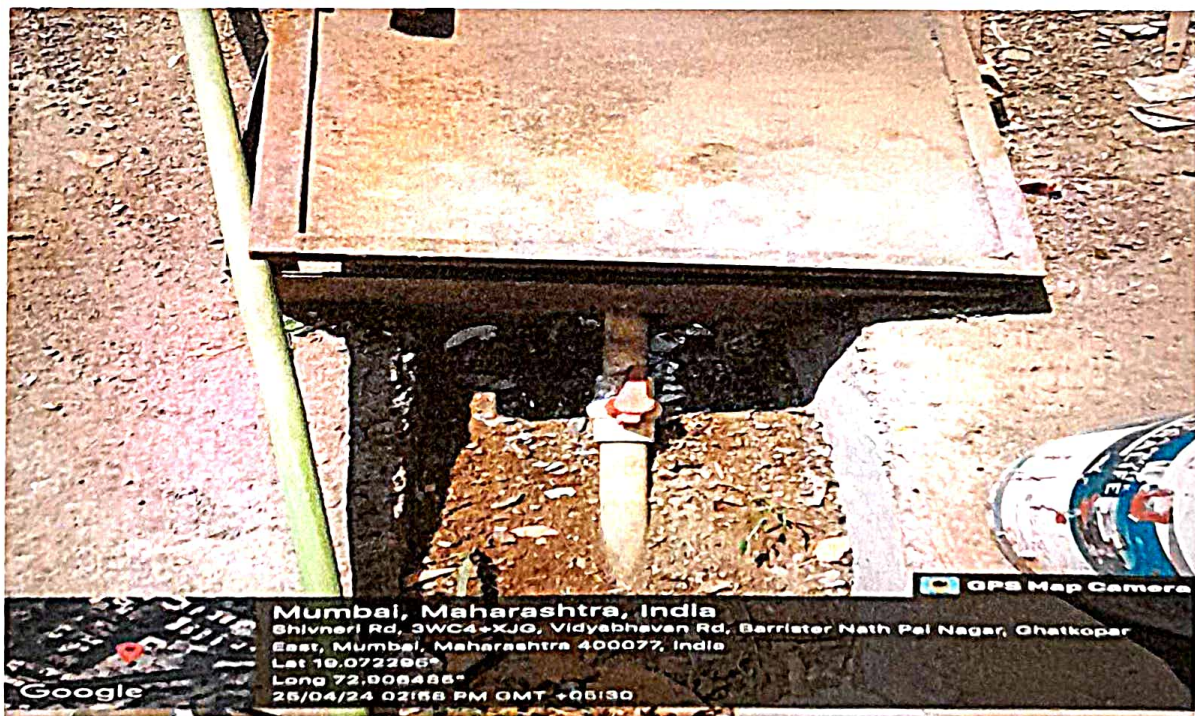
BMC water inlet for both drinking water tanks and multi-purpose tanks
